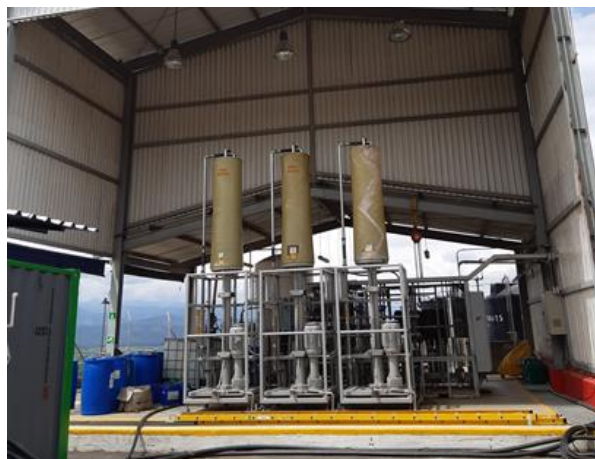
Foto 37. Reactores VSEP (Vibratory Shear Enhanced Process)
