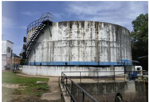
Reactor – Filtro Percolador
