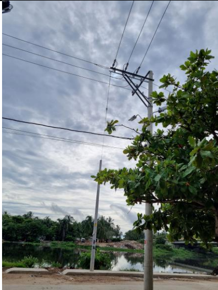
10°59'21.5"N 74°46'36.1"W, Estructura fin tramo 2 conductor AAAC 246,9. 210 ml.
