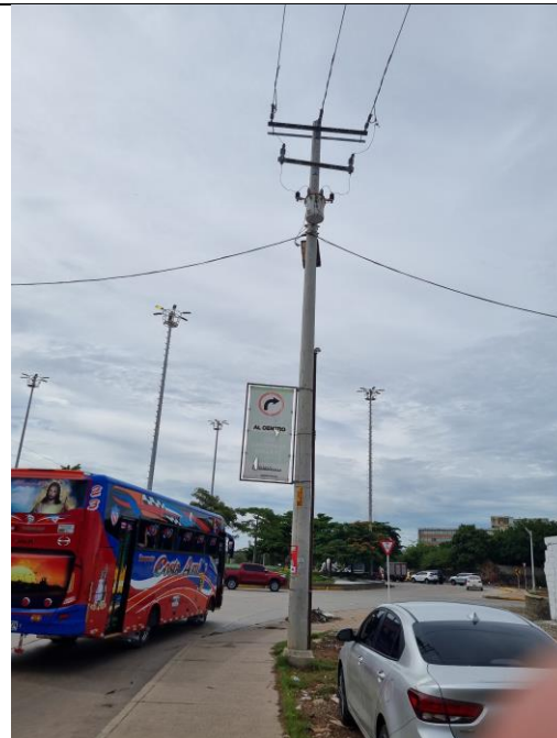
10°59'16.9"N 74°46'39.2"W, Estructura terminal tramo 6, conductor AAAC 246,9 244 ML
