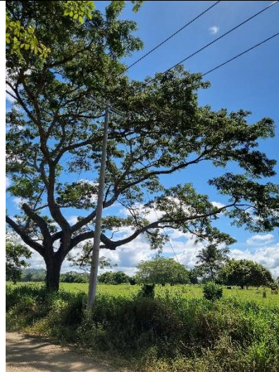
8°43'13.9"N 75°57'04.6"W, Estructura intermedia cambio conductor a CF125.
